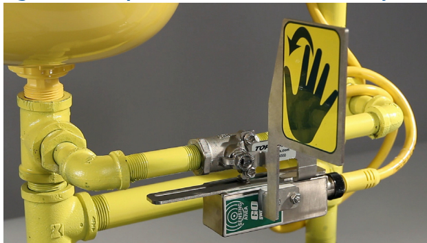
Figure 7-17. TopWorx Switch Installed on an Eye Wash Station.
