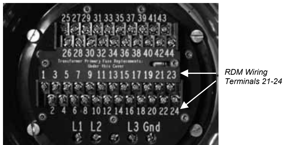
Figure 3-22 Connecting RDM Cables to the STC
