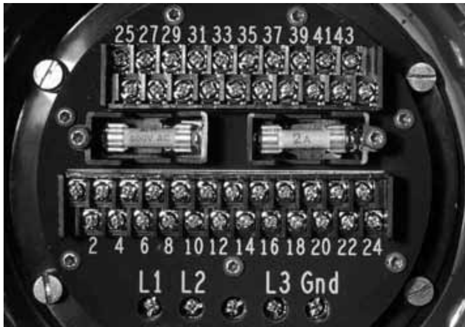
Figure 7-1 Fuses in the STC
