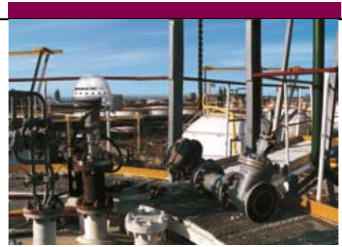
Installation of TankRadar Rex with the tank in service.
