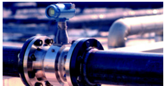
The Rosemount 8800 Series Vortex Flowmeter Installed
