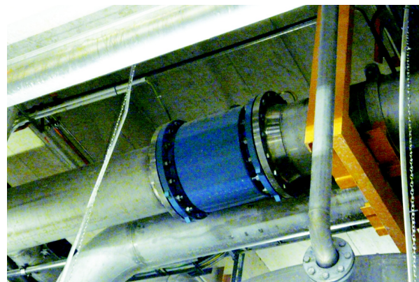
Rosemount 8700 magnetic flowmeter installed
