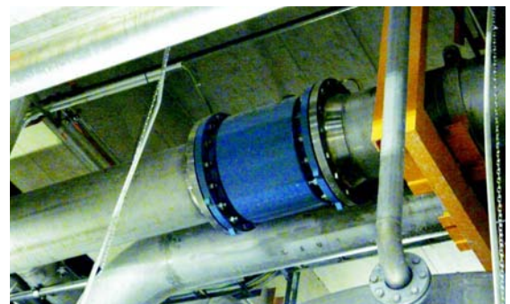
Rosemount 8700 magnetic flowmeter installed
