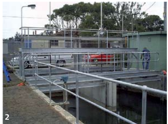
Figure 1 Two 3100 transmitters mounted on 5" diameter 316 stainless steel stilling tubes.
