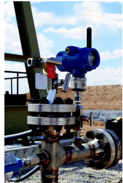
The Rosemount 3051S Wireless Pressure Transmitter Installed
