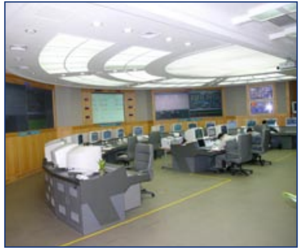
The main control room at the Yonghung Power Plant allows operators to view information pertaining to any process in the plant.
