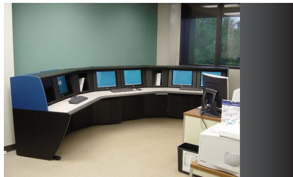
The Scenario solution for Dairyland's J.P. Madgett station mimics the control room layout to provide realistic training conditions for the plant operators.
