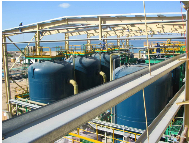
Dual media filters at the Ghalilah Ras al Khaimah Desalination plant.
