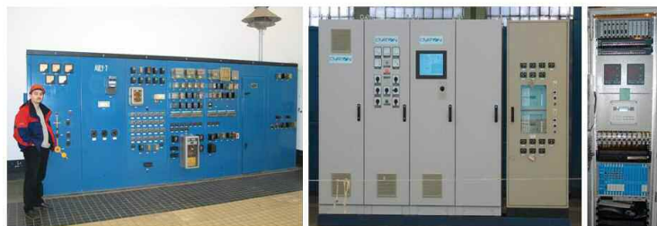
Volzhskaya 8 was the first unit to undergo modernization by Emerson. Obsolete cabinets (far left) were replaced by Ovation controller cabinets (center). The inside of one Ovation cabinet is shown on the far right.
