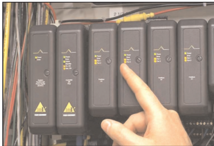
Photo 1. Portion of the Emerson DeltaV™ controller running the new dye skid at FiberMark, Brattleboro, Vt. Shown (left to right) are the controller's backplane-mounted power supply card, CPU card, and four FOUNDATION™ fieldbus communications cards having two fieldbus segments each. Fieldbus instruments provide almost all analog functionality. The integrated DeltaV digital automation system is a key component of Emerson's PlantWeb® digital plant architecture.
