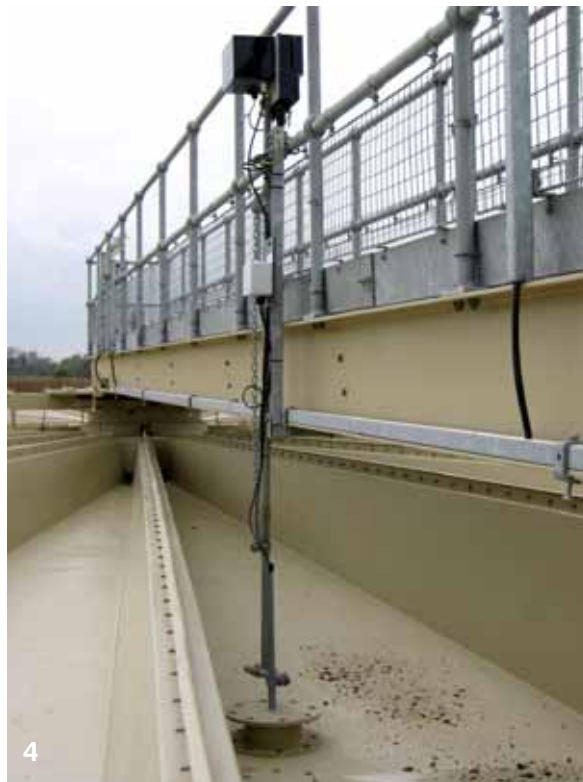
Figure 4 MSL600 installed on the settlement tank
