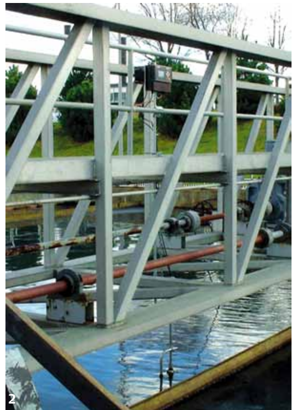
Figure 1 Highland Creek treatment works Figure 2 MSL600 installed over the primary settlement tank
