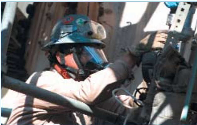
Figure 4. Hot cutovers of transmitters required only the repositioning of process measurement tubing from old to new.
