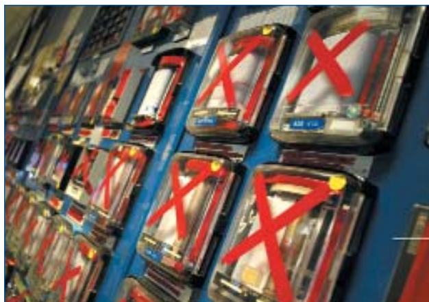
Figure 5. Red tape over old control panel gauges reminds operators as each loop is shifted onto the new quad console.
