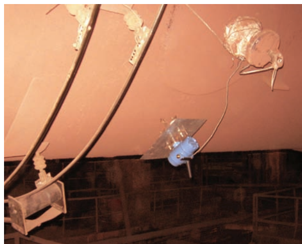
Rosemount 648 Wireless Temperature Transmitter connected to the kiln's existing thermocouples on a heat-proof ceramic seal.
