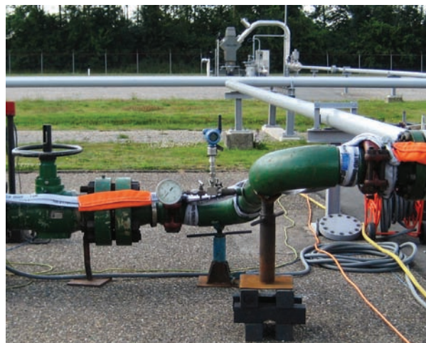
Emerson’s wireless sensors are used by NAM to measure differential pressure and temperature as part of a mobile well head test system.
