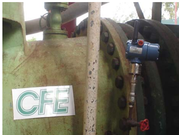
CFE LAPEM uses Smart Wireless transmitters for temporary measurement.
