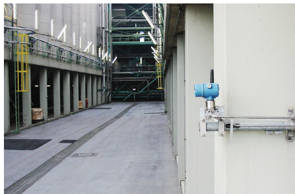
Eight Rosemount 3051S DP wireless transmitters were installed at the INEOS plant in Cologne.
