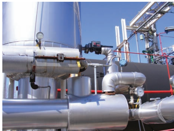
The Fisher 4320 wireless position monitor installed in the Ethylene Oxide unit is about twelve feet off the ground.
