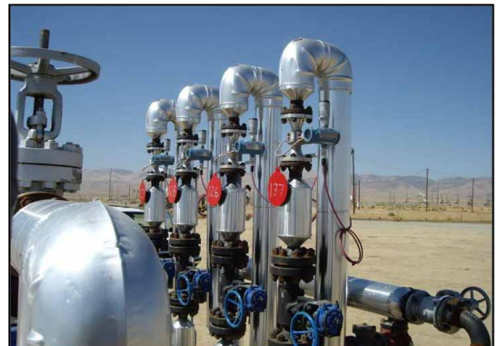
A ball trap connected to a turbine meter was used to measure oil flow from one of seven producing oil wells on any given header. A Rosemount 8800 MultiVariable vortex meter with a WirelessHART THUM now provides a low-maintenance option that gives continuous, one-minute updates for each individual well.
