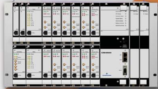
Online Machinery Monitoring
