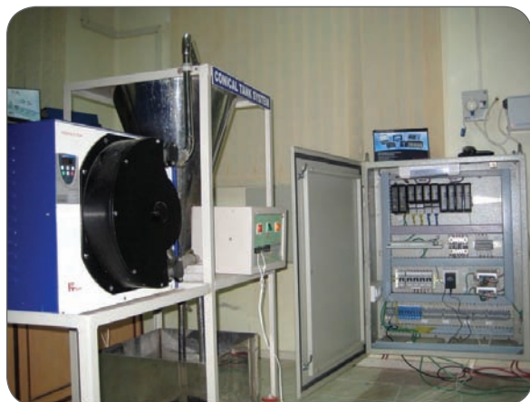
Figure 1. Conical Tank in MIT Anna University Lab with an industrial DCS.
