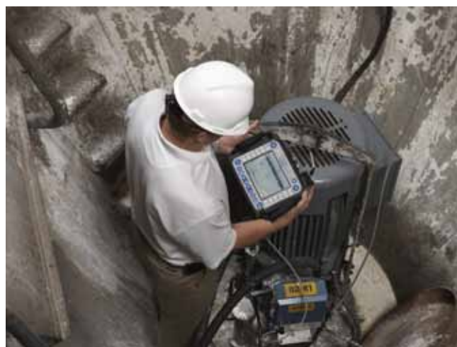
Using a machinery health analyzer to retrieve spectral data files captured by the continuous vibration transmitter at the Elk River Station. Photo, Novaspect Inc.
