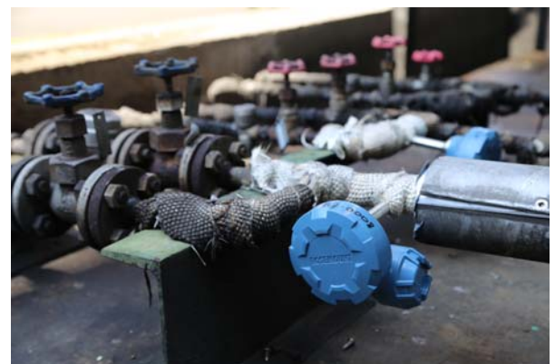
Rosemount 708 Wireless Acoustic Transmitters installed on the steam traps
